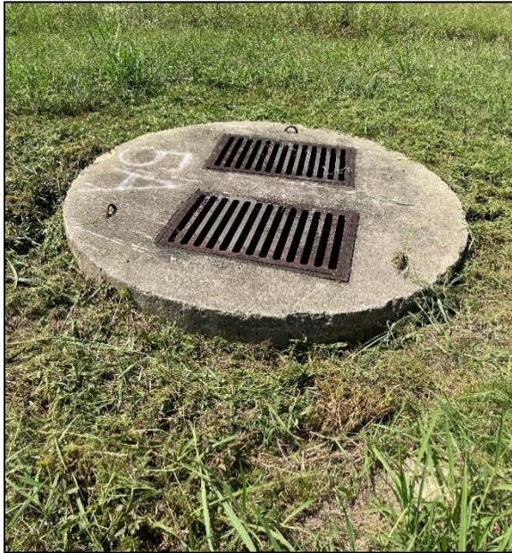
Erosion at Inlet
