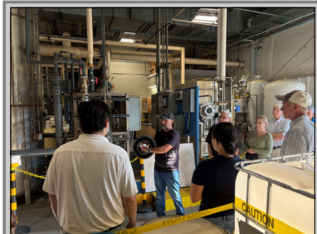
Mr. Humberto Altamirano discussing the dual-walled pipe used to convey extracted groundwater and leachate from LF003 to the GWTP.
